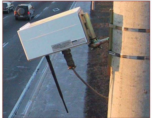
RTMS (Remote Traffic Microwave Sensor) radar
